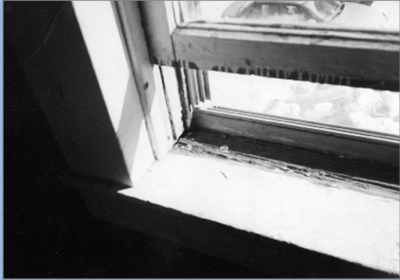
A window well with deteriorating lead paint—a common site for lead poisoning.
